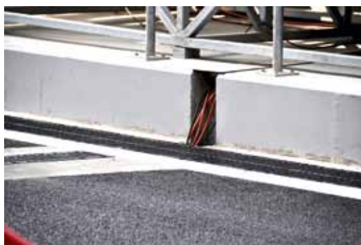
At Yas Marina Circuit in Abu Dhabi the HAURATON SERVICE CHANNELS are used in the pit lane
