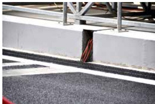
At Yas Marina Circuit in Abu Dhabi the HAURATON SERVICE CHANNELS are used in the pit lane
