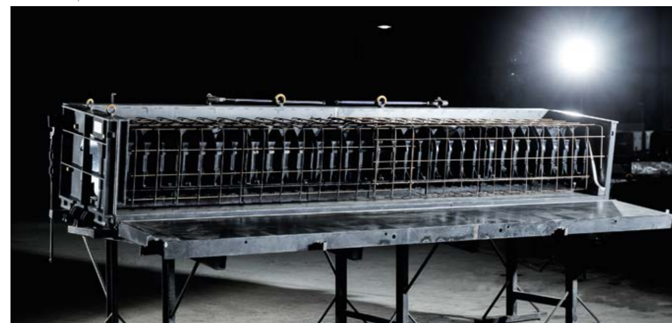
Form with drainage elements and reinforcement, ready to be poured with concrete
